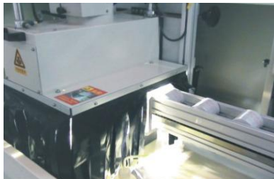
UV Curing System
